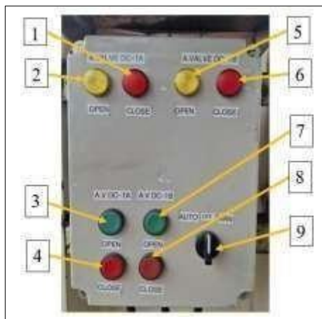
Gambar 11. Sistem Panel Kontrol Motorized Valve
