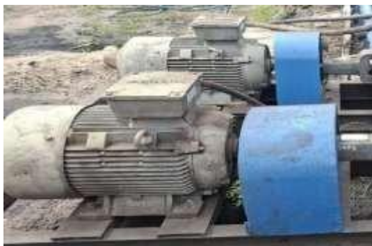
Gambar 6. Motor Pompa Chemical
