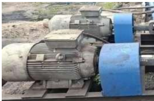
Gambar 6. Motor Pompa Chemical
